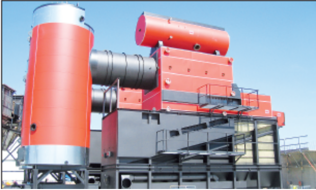
Weiss A/S boiler working on solid domestic waste
